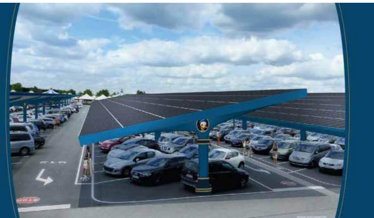
The Disneyland Paris solar canopy, shown above, broke ground in FY20.
